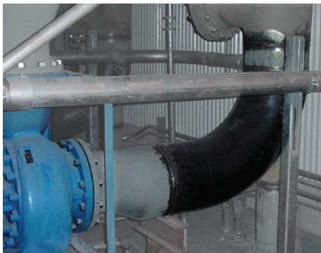
Vortab VEL installation at pump inlet
